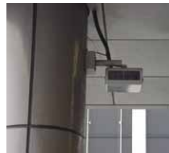
AXIS Q1755 in the original PMC housing, installed facing the entrance to the parking lot.
