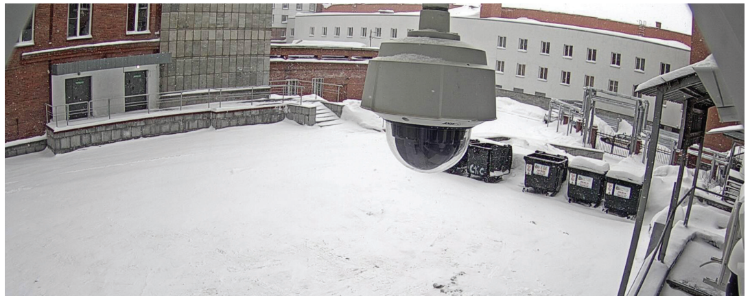
Figure 6: Axis test camera installed on site in Novosibirsk.
